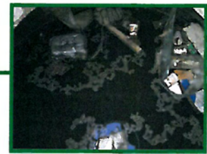
Standing Water is Not Clear & Bacteria Growth Visible.
